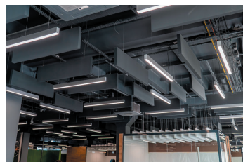
Acoustic baffles compete with light fixtures for space and their own piece of the budget resulting in compromises and clutter.
